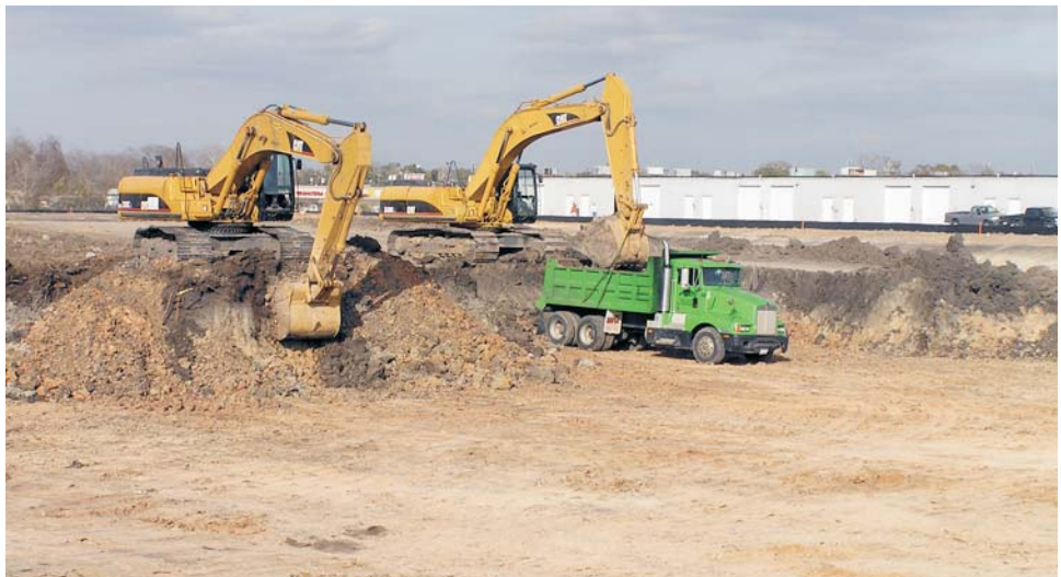
Construction continues with work on the Willow Waterhole Stormwater Detention Basin. Once Phase 2 is complete, 700 acre feet of stormwater storage will be added.
