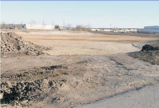
Hundreds of thousands of cubic yards of dirt are moved from each detention basin project. So where does the dirt go?
