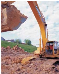
Progress continues on the stormwater detention basins at Arthur Storey Park where construction is estimated to be completed in 2009.
