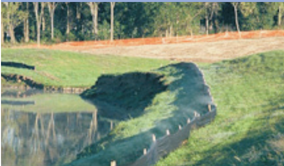
Site preparations began in September 2004 for the Freshwater Tidal Marsh Project located at Mason Park.
