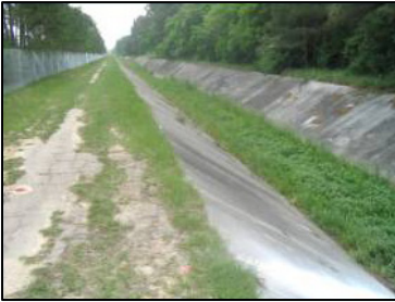
Sediment accumulation on HCFCD Unit K149-00-00.
