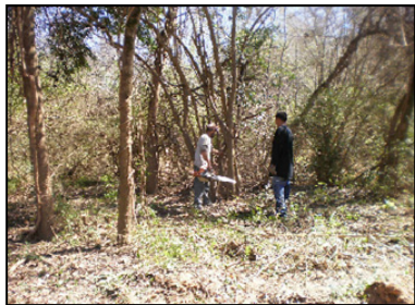
Selective clearing on a tributary of Unit P114-00-00 looking downstream of Unit P114-01-00.
