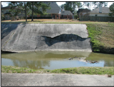
Concrete slope paving failure on a lateral of Rogers Gully (Unit G103-24-03) at the confluence of Rogers Gully.
