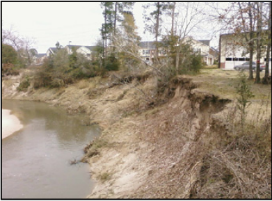
Erosion along the channel bend of Cypress Creek at Klein Fire Station.
