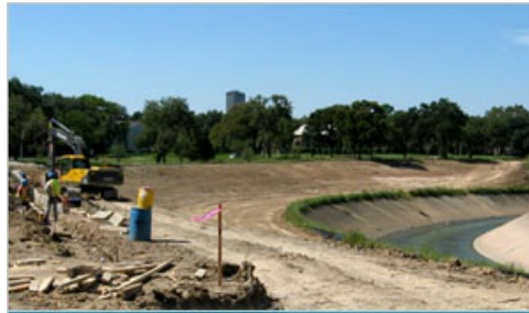
One of the largest construction phases to reduce flooding from Brays Bayou began on June 21, 2010.
