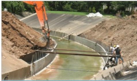
Repairing the concrete channel lining reduces the possibility of future concrete lining failures.
