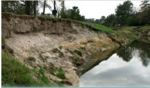
After repair is complete, native grasses will be established along the slope to help prevent future erosion.
