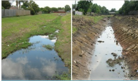
Before and after photos showing repairs on a tributary of Turkey Creek paralleling Grapewood Drive.
