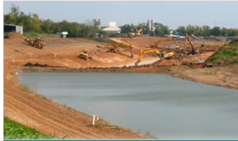
Starting from the Houston Ship Channel, more than 19 miles of bayou widening and deepening will be completed by 2012.
