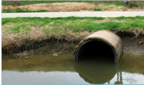
Storm sewers are maintained by local cities or municipalities, but this storm sewer in Shoreacres is an exception to the rule.
